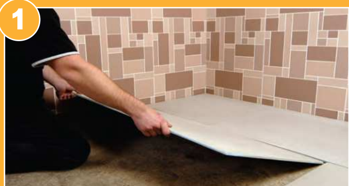
1. Fit the JACKBOARD Insulated Tile Backer Board to the floor securely following the manufacturers instructions.
