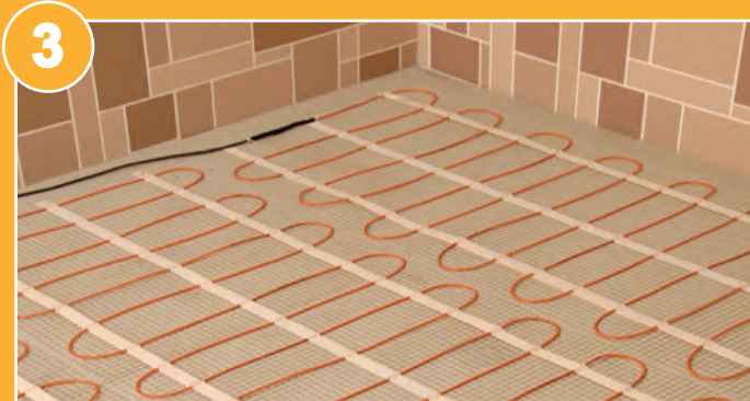
3. When satisfied with the proposed layout fix the matting to the floor using the integral self-adhesive fixing strips.
